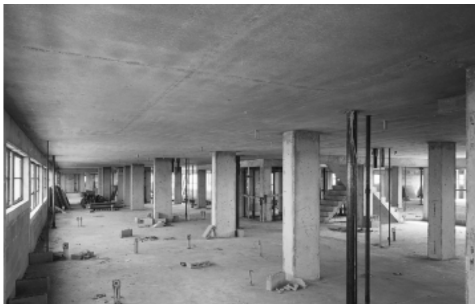
FIGURE 1.3 Flat plate floor slab, carried directly by columns without beams or girders. ( Portland Cement Association. )
