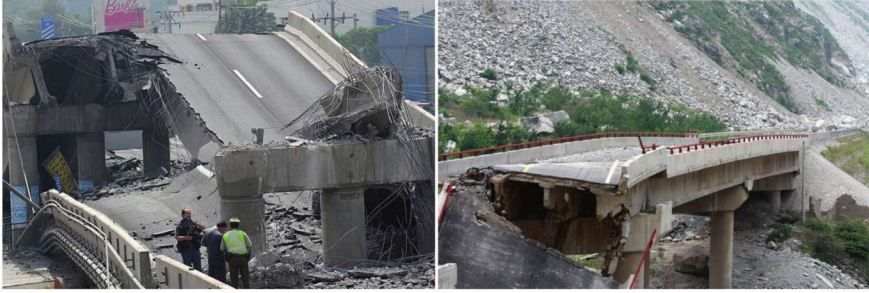
Fig. 1.2 Damage of bridges
