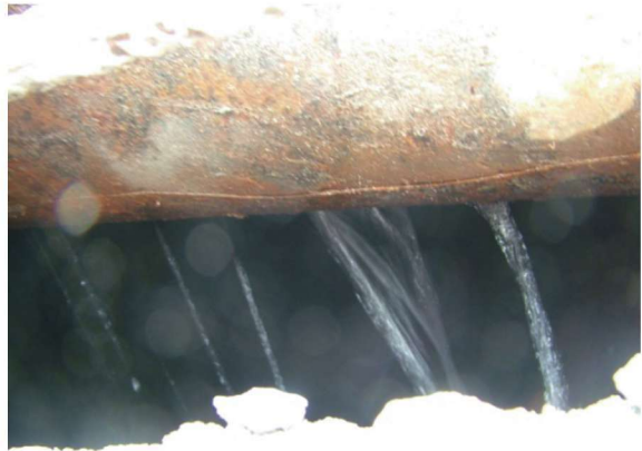
Fig. 1.6 Crack of the pipe
