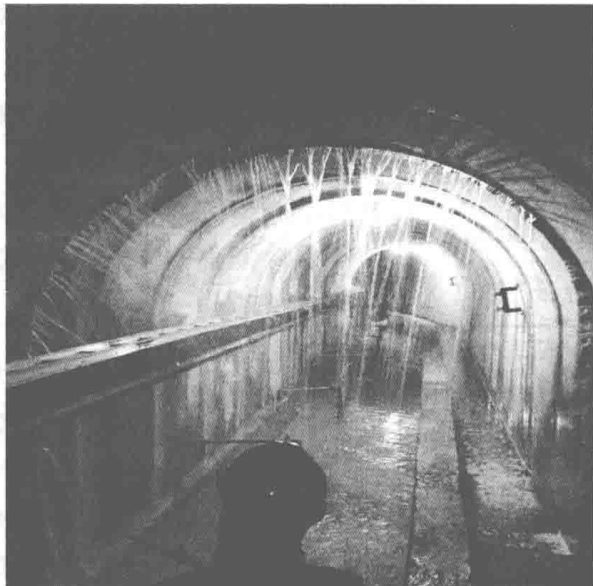
图4 EL. 1002m(1号纵向排水廊道)裂缝漏水情况
