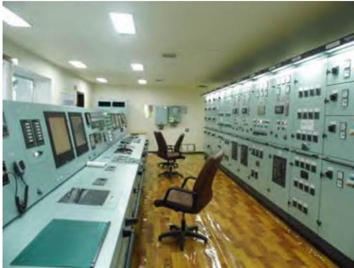
Fig.1-4 Engine control room(ECR)
