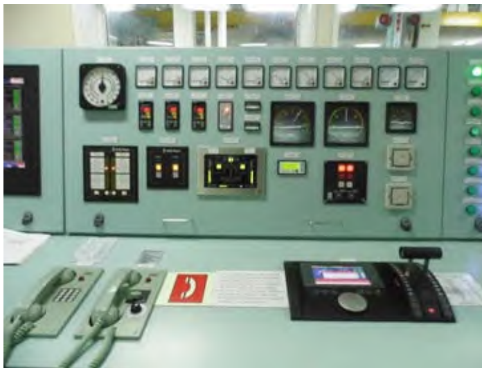
Fig.1-5 Engine control console(ECC)
