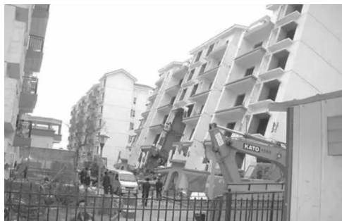
(a)温州楼房倒塌
