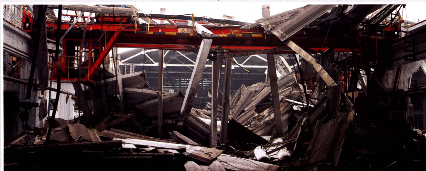
▶ 攀长钢四厂受损严重的车间
