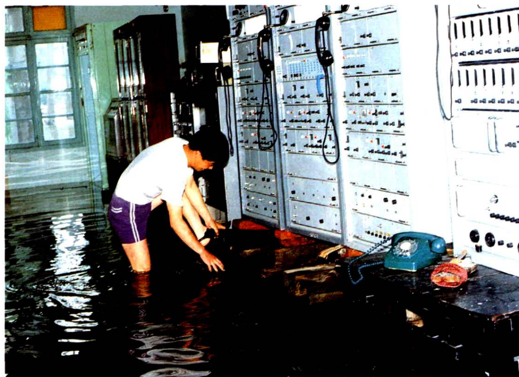
胥门变电站及相邻的载波室受淹情况(1991)
