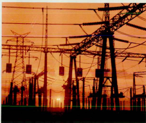
大坝发电厂开关站一侧
