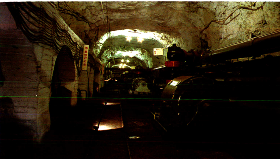
-580水泵房 - 580 Compressed Water Pump Room
