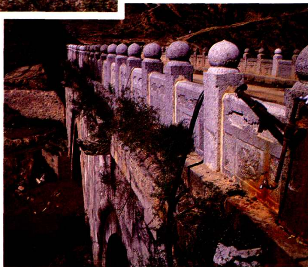
三原龍橋——明萬曆三十年（1602年）建成。 Lung (Dragon) Bridge in Sanyuan—built in 30th year of Wanli (1602), Ming Dynasty.
