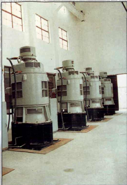
城市防汛排涝泵站 Urban drainage pumping station
