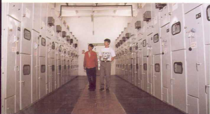
轮南联合站燃气发电站高压室 Hyperbaric chamber of gas generator centre in Lunnan joint station.
