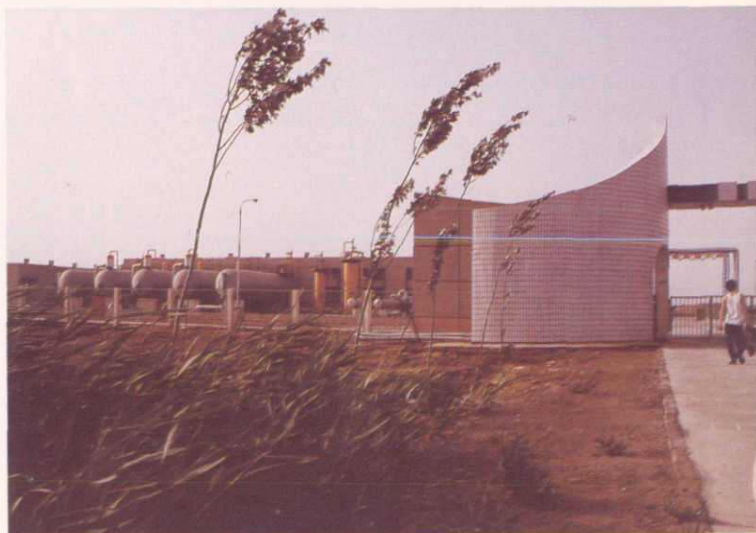
桑塔木油田集油站 Oil gathering station of shangtamou oilfield.
