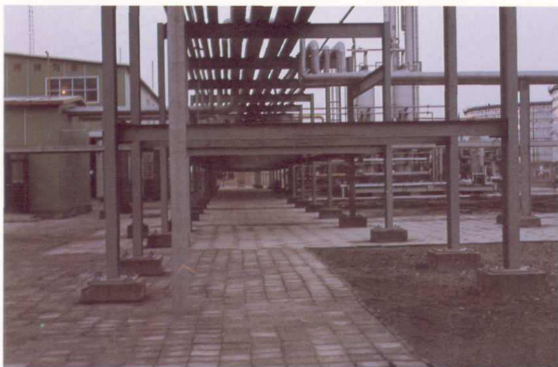
轮南 20 万吨轻烃站一角 A corner of 200,000 Ton lighter hydrocarbons station in Lunnan oilfield.
