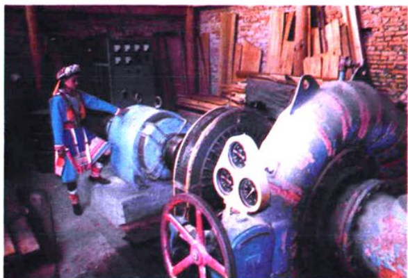
腾冲县古永乡寨桥电站机房
