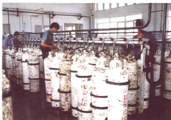
溶解乙炔厂充罐车间
