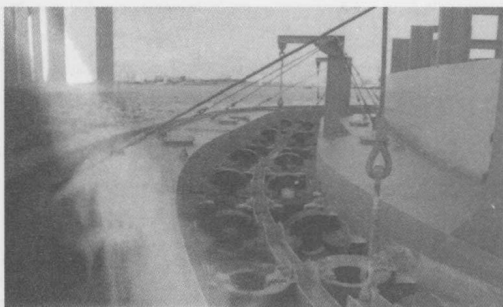
a) 广东湛江海湾大桥主塔柔性防船撞装置 The soft anti-collision equipment at the main tower of Zhanjiang Bay Bridge, Guangdong province
