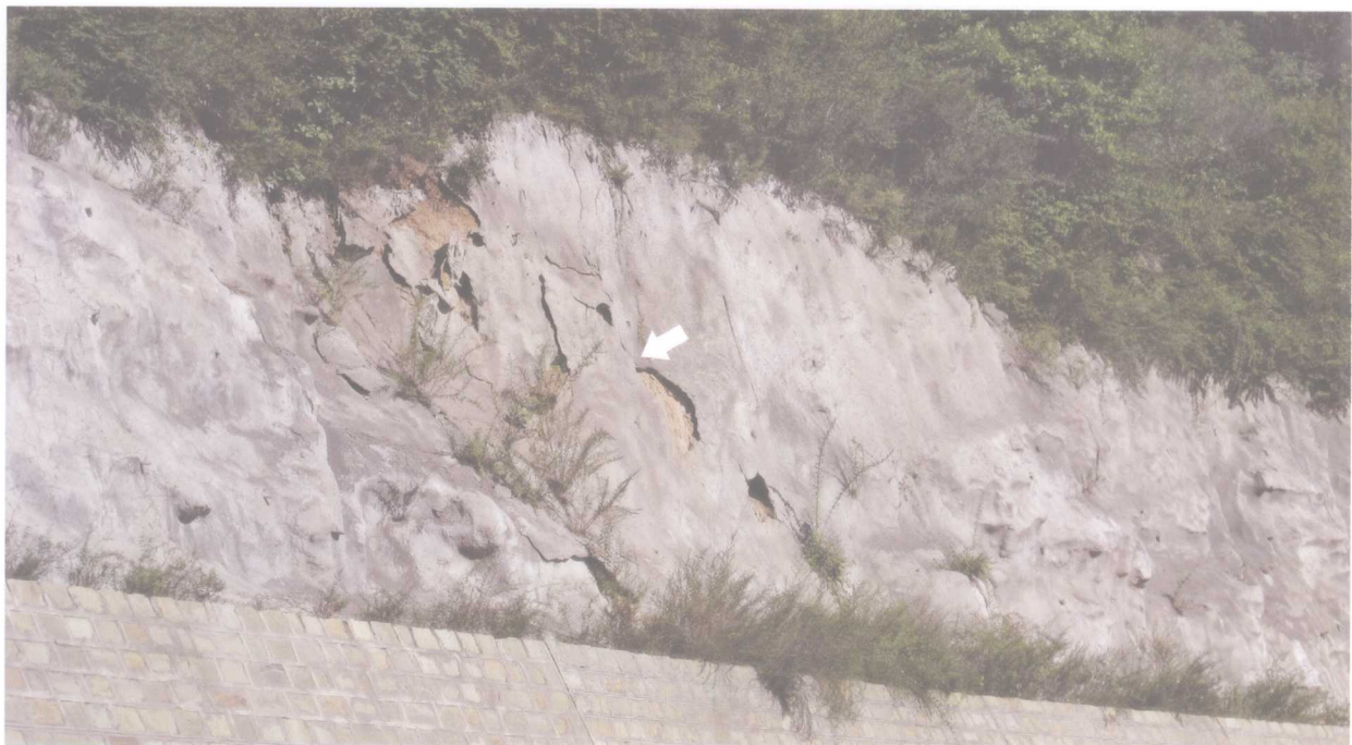
② 局部剥落 Localized collapse
