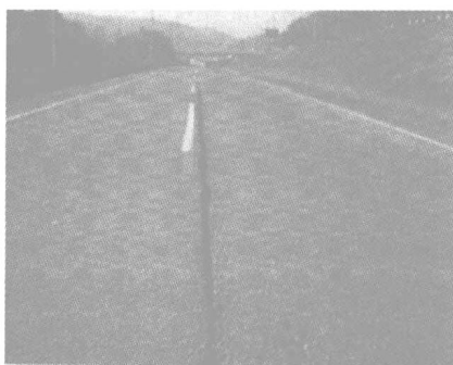
(k) 纵向裂缝
