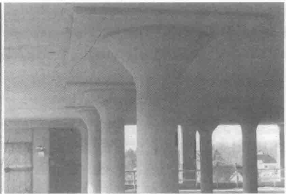
Fig. 1-4 Flat slab floor, without beams but with slab thickness increased at the columns and with flared column tops to provide for local stress concentration of forces.
