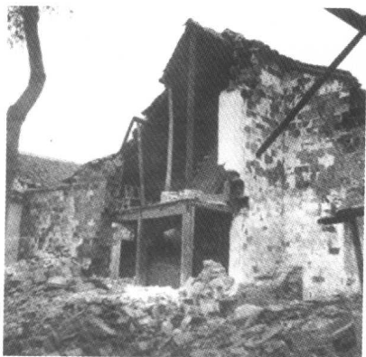
1. 溧阳上沛两层薄砖空斗墙墙体垮落,木柱歪斜
