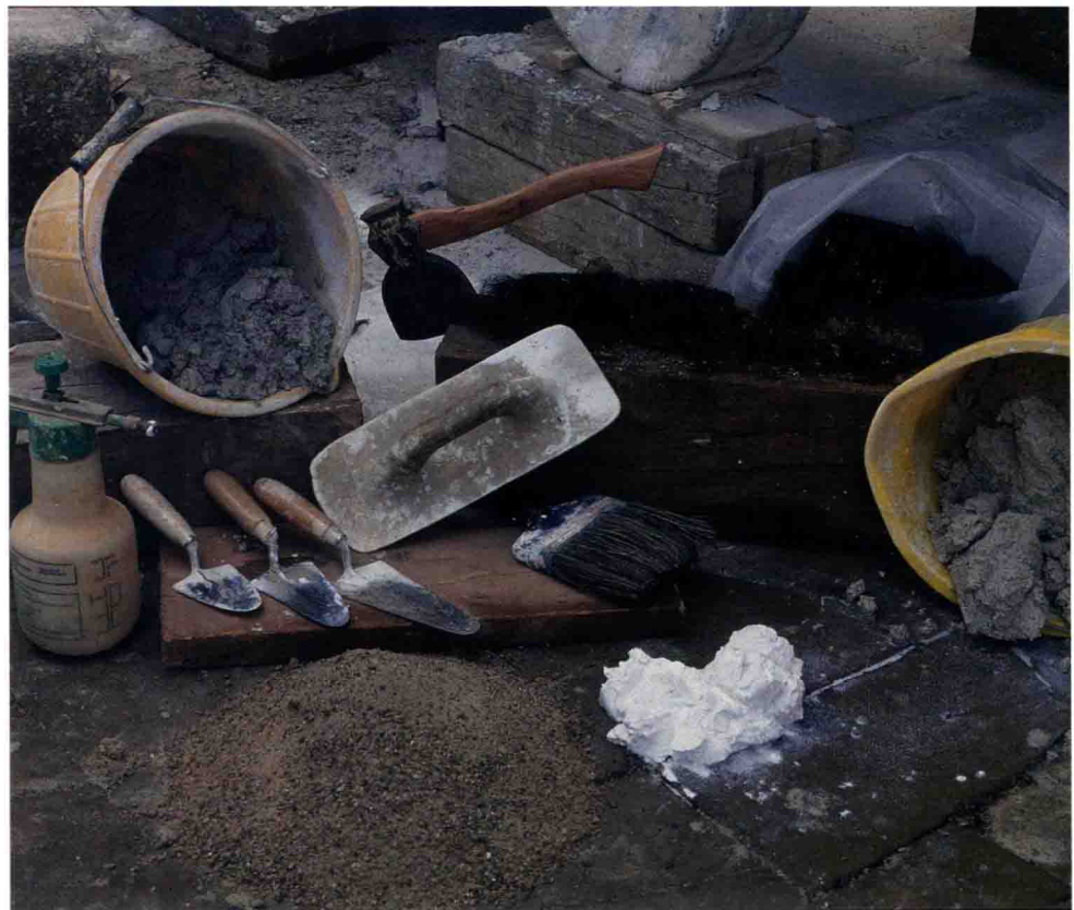
The lime revival was driven not only by pragmatism, but a fervent belief in the craft of lime.
