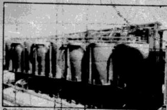
Precipitation unit 沉淀槽
