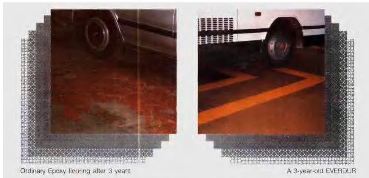
Ordinary Epoxy flooring after 3 years
