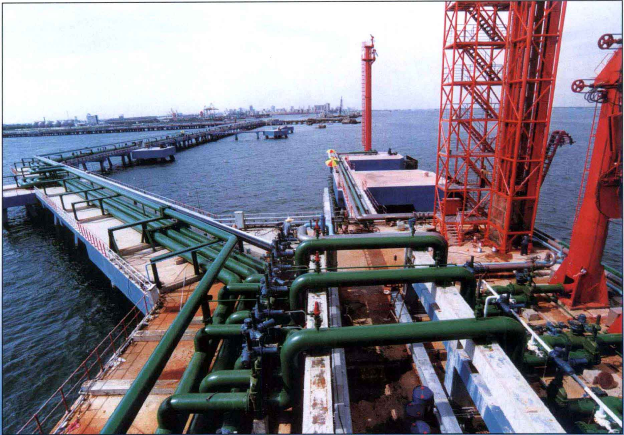
■ 30万吨级油码头 300,000-ton oil Terminal
