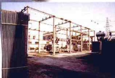
变电所 The transformer substation
