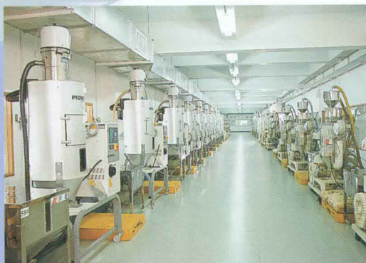
Plastic Resin Drying & Handling System
