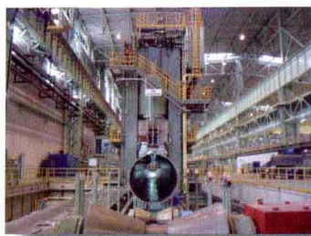
世界领先技术装备水平的油气专用直缝焊管UOE机组技术集成项目 Straight welded pipe for oil and gas at nowadays highest technical furnishment level for UOE Unit technology Integration Project
