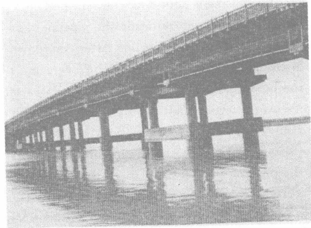
Fig. 4. The Luning pipeline crossing Huaihe river, with one pipeline at each side of the lower bridge
