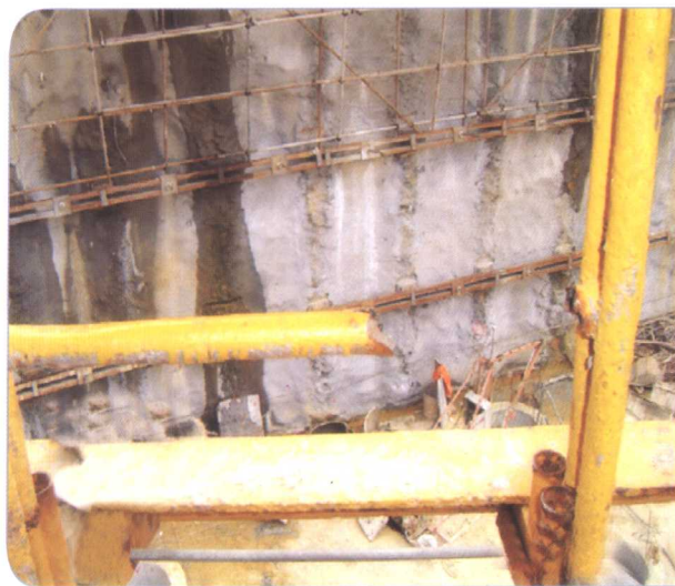
爬梯横杆断裂
