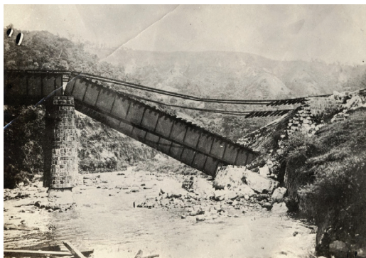
地震中坍塌的桥梁
