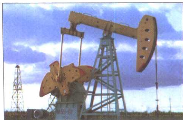
肇东市储油罐和采油井
