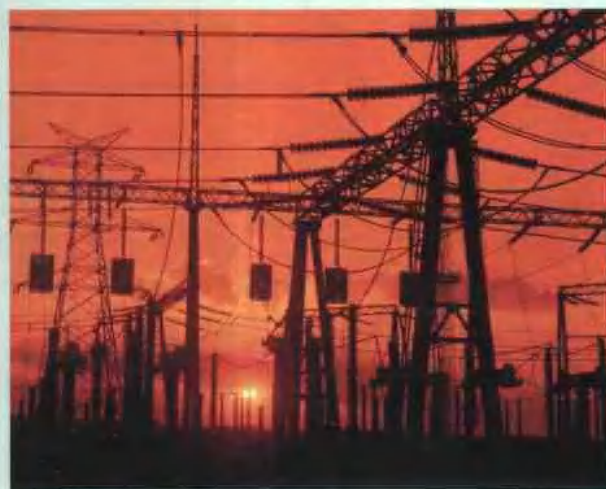
大坝发电厂开关站一侧
