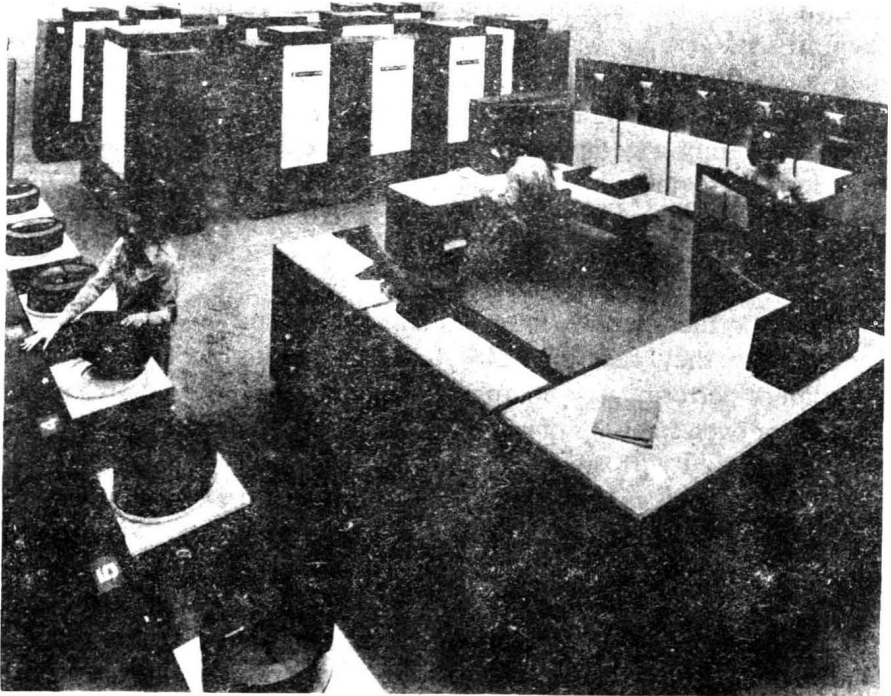
A bank of computers and other components in a modern computer installation. (Courtesy Honeywell, Inc.)
