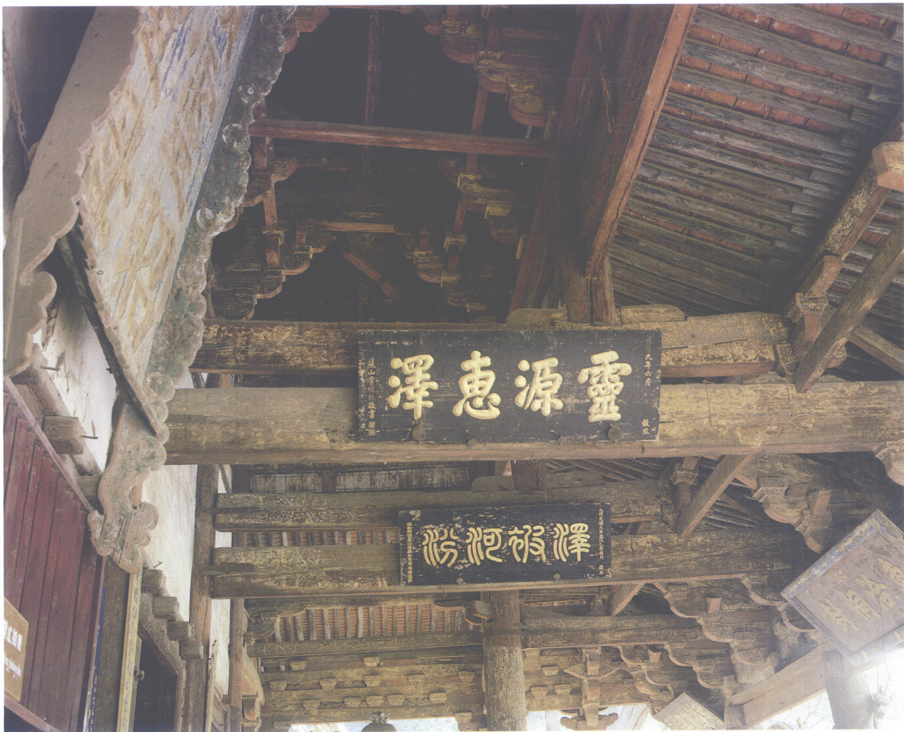
晉祠聖母殿前檐結構 The front of the Hall to Holy Mother
