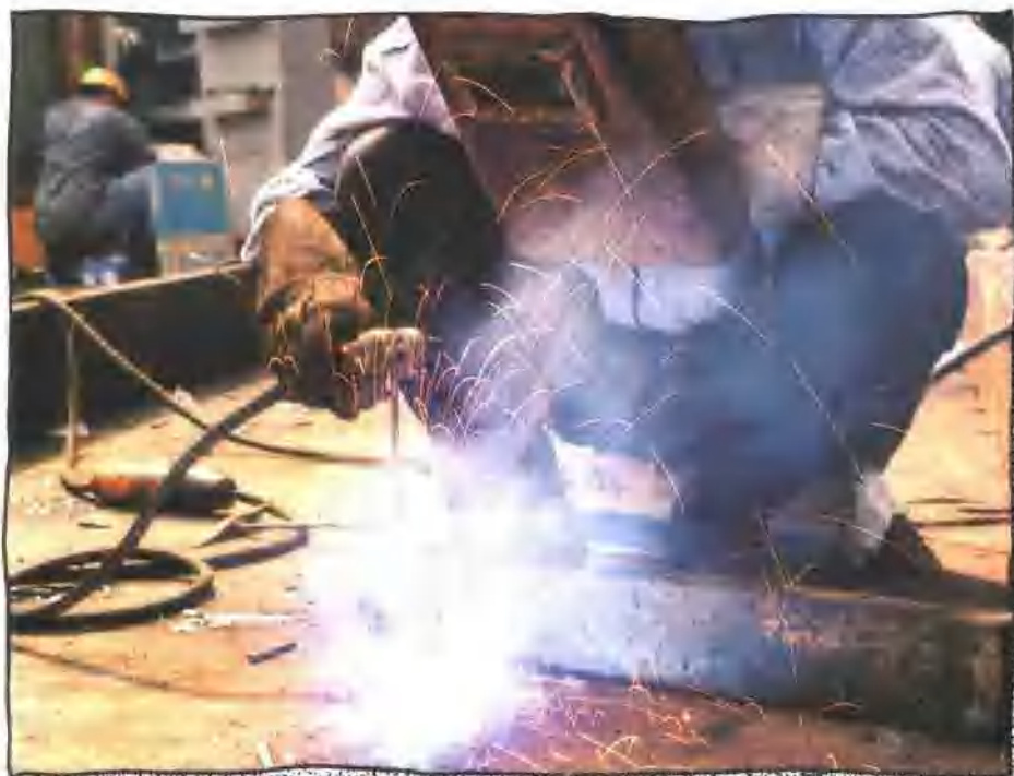
Welding may generate metal fumes and toxic gases.
