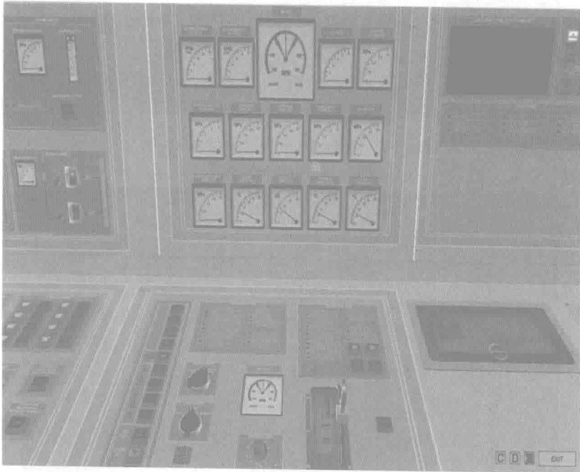
Fig. 1-9 Engine Room Control Station(ECS)
