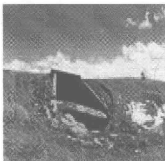
(b)输水涵渠的基础冻胀变形破坏
