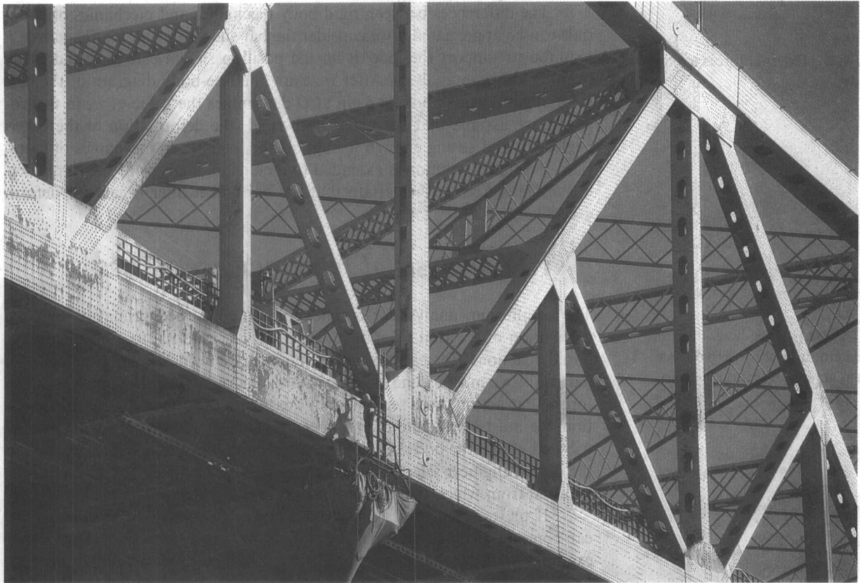
Truss of a highway bridge. The members of a truss carry loading by direct tension or compression; there is very little bending. A truss is an efficient structure in the sense that it has a high load/structural weight ratio.
