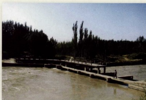
◎ 胜利渠分水闸
