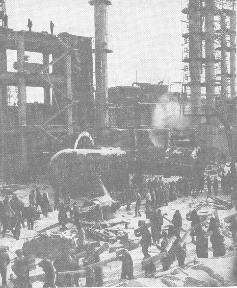
Displaying their glorious hard-working tradition, Taching people putting up new installations for the multi-purpose use of petroleum.
