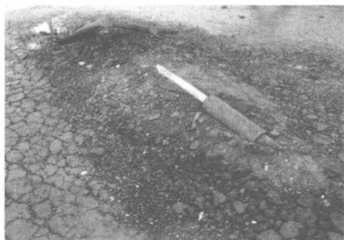
(c) 冻胀拔起通信电缆
