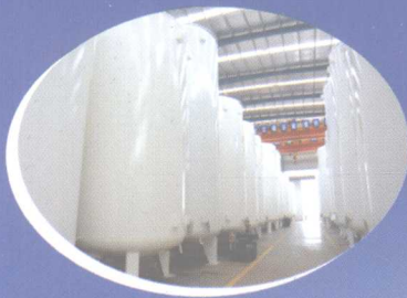
低温液体贮罐
