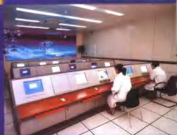
甘肃电信网管中心 The networks management center of Gansu Provincial Division of China Telecom Group Co.ltd
