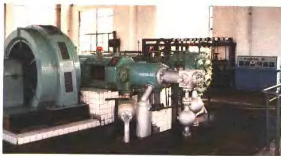
⑯化肥厂压缩车间
