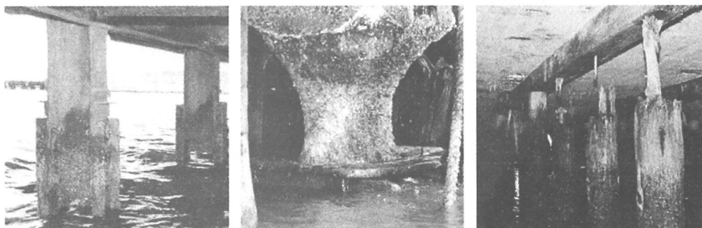
(a) 腐蚀的钢桩
