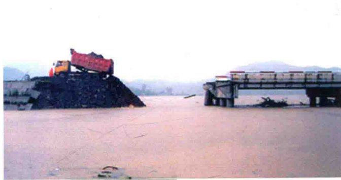
灌水、长甸镇多处公路桥被洪水冲毁
