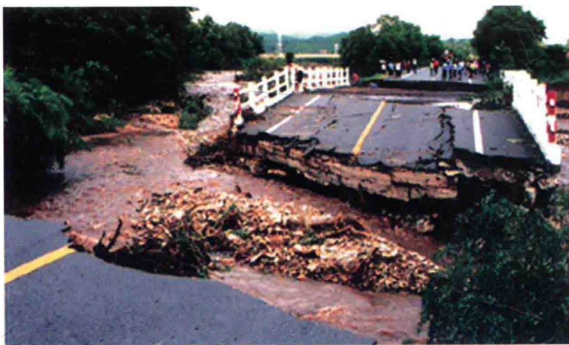
灌水、长甸镇多处公路桥被洪水冲毁
