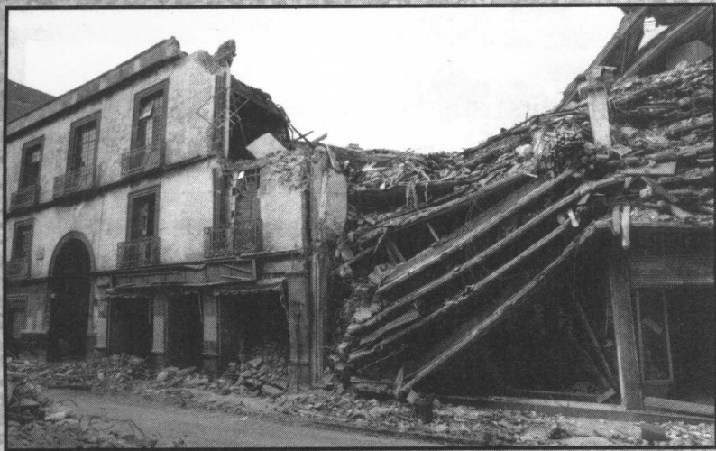
After an earthquake in Mexico City
