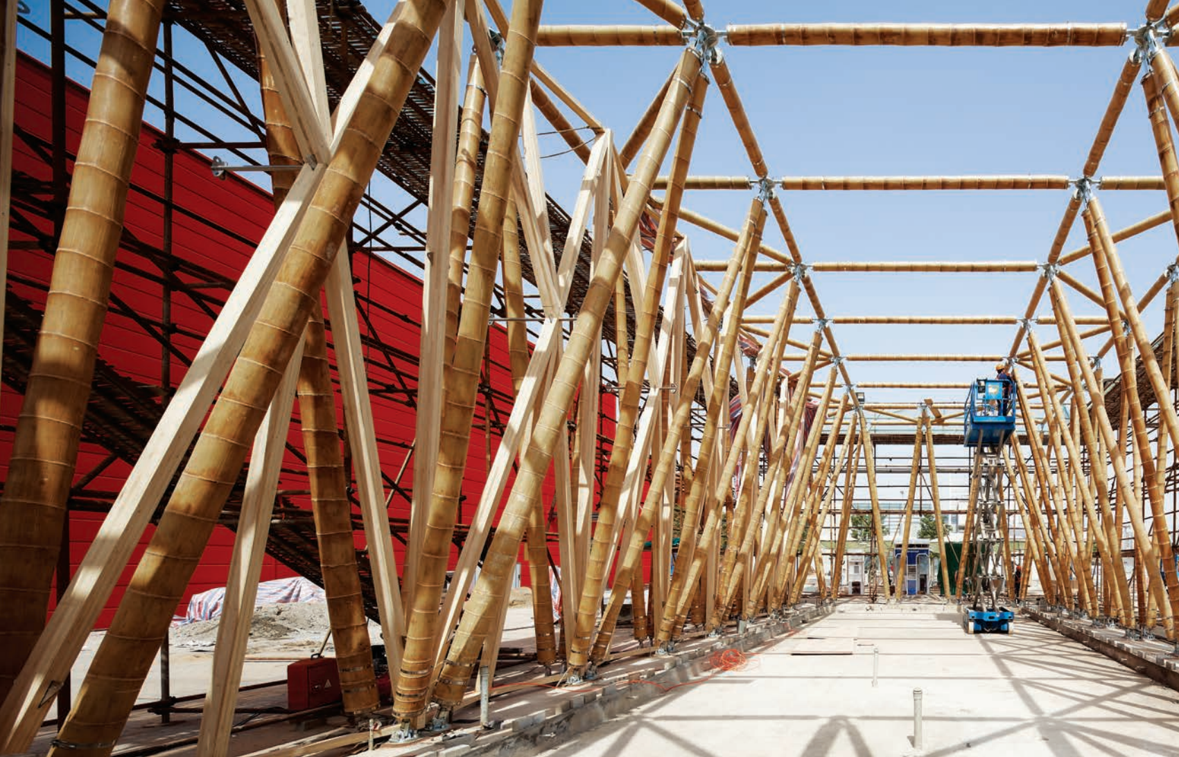
带螺栓的竹压板外立面框架、竹杆构成的V形主体结构 Bolt-on connection of the bamboo-laminate beam facade and V-shaped main structure made of bamboo rods
