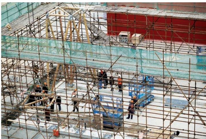
为德中同行之家展馆树立起的第一组竹支撑柱 Erecting the first bamboo supports for the German-Chinese House
