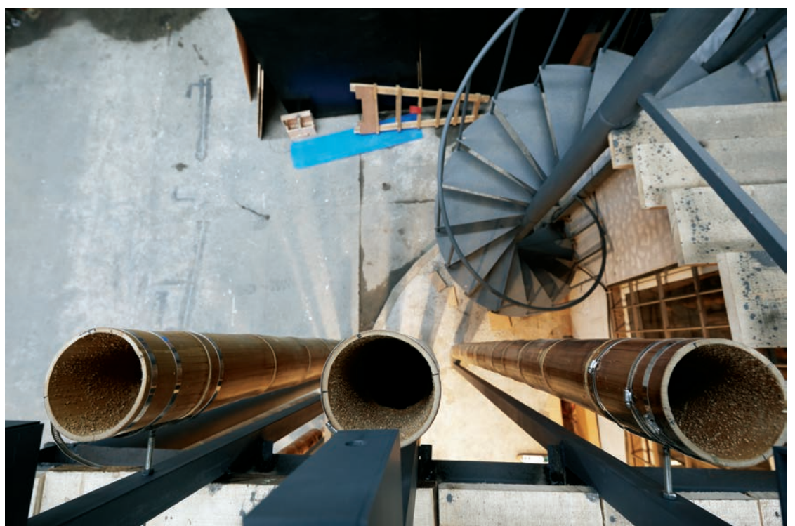
预先组装的由钢制连接件及特殊配比混凝土 加工处理的竹杆 Pre-assembly of the bamboo rods with connecting elements made of steel and special concrete
