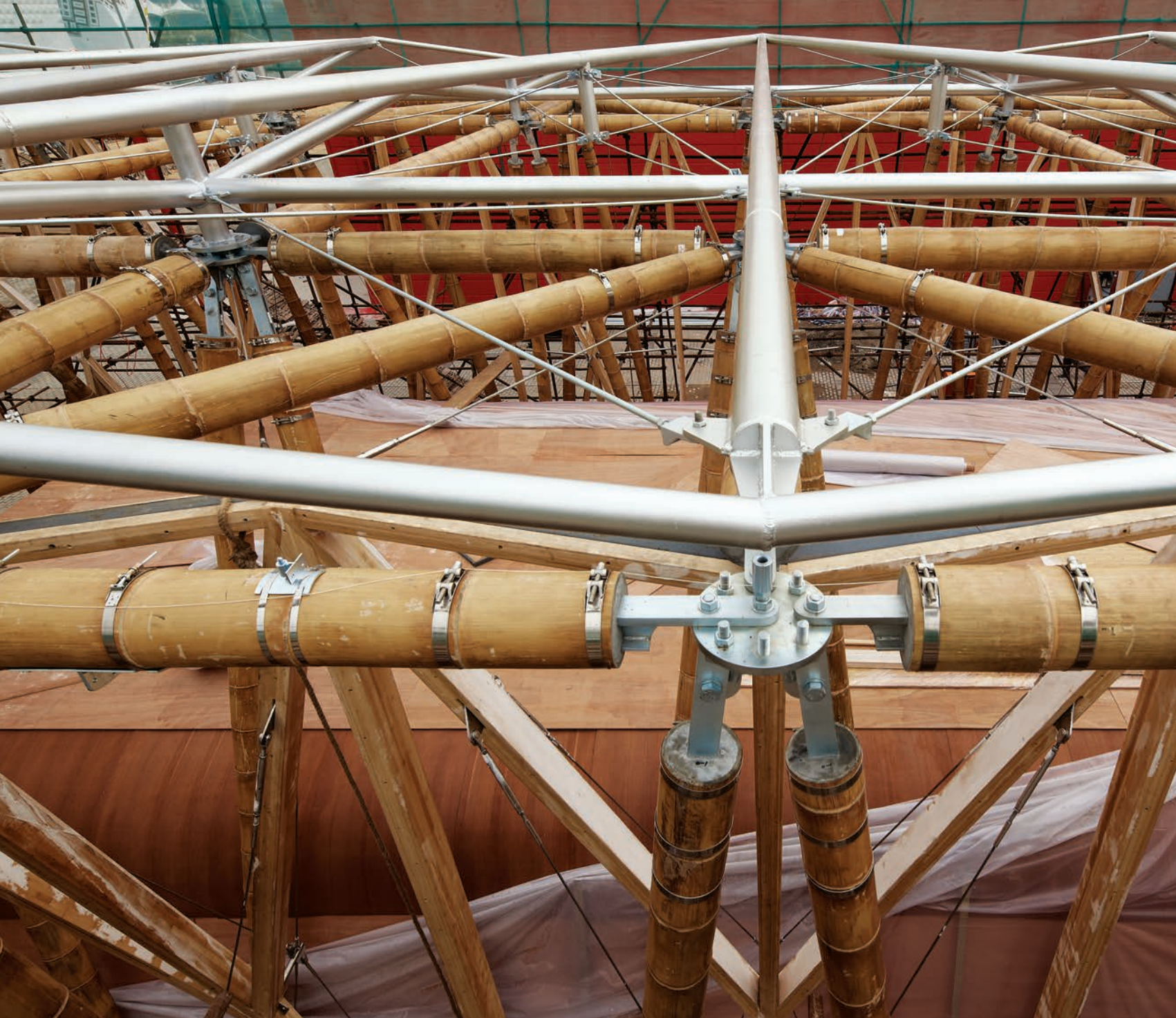
处于基础搭建阶段的顶部节点 Roof nodal points in the foundation during construction
