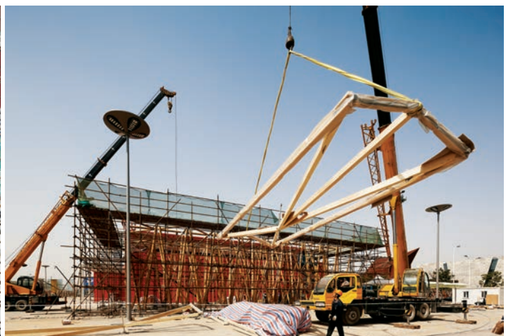
搭建过程——组装构成外立面的竹压板条 Assembling a facade element made of bamboo laminate
