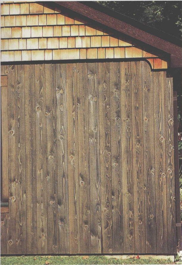
WA-15 山墙上装有新的杉木的垂直木镶板，住宅车库 Vertical board siding with new cedar shakes on gable, residential garage
