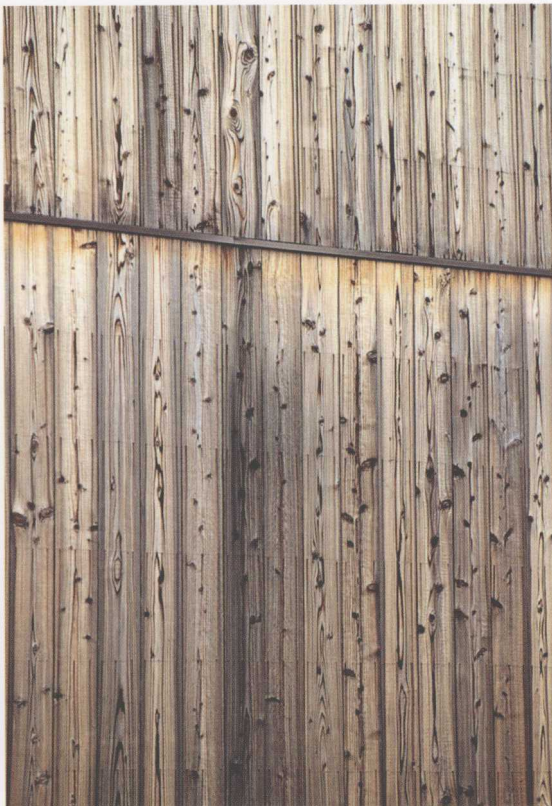
WA-7 多层杉木的齐平弦切板墙，配有水平分割板条 Knotty-cedar flush, vertical plain-sawn board wall, with horizontal batten divider
