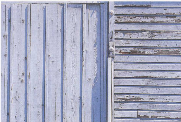
WA-11 喷漆风化木镶板，左：木板和板条；右：隔板 Weathered painted wood siding. Left: board-and-batten; right: clapboard
