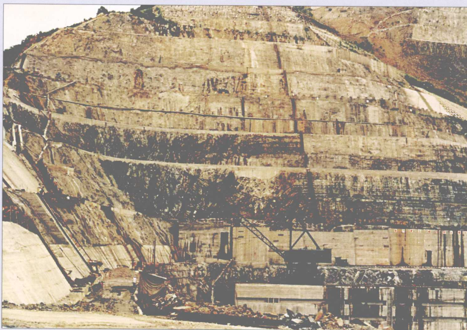
图1.5 正在施工中的厂房西坡 Fig. 1.5 The west slope of the plant under construction
