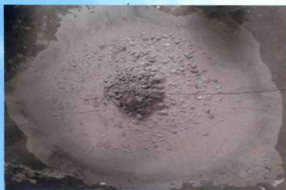
出现严重离析的混凝土 Serious segregation of concrete
